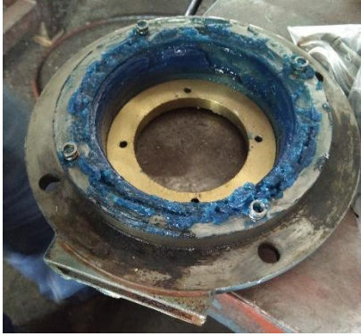
Fig. 14 – Old hardened grease in bearing cap
